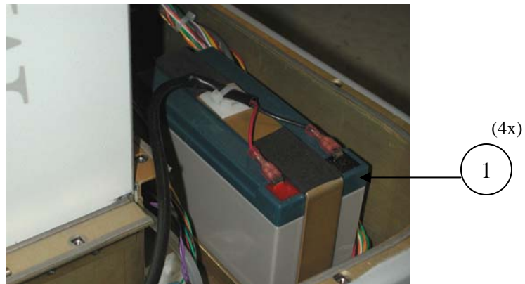
Figure 2: 3150M, View of Base, Battery
