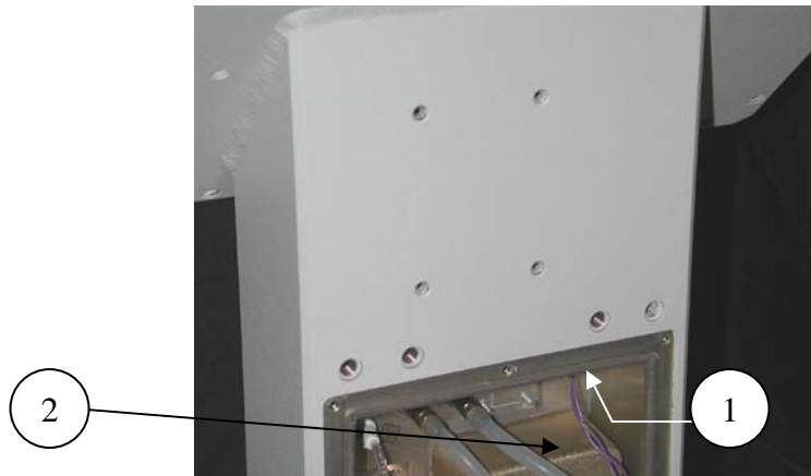
Figure 3: 3150M, View of Column, Fiber Optic Cable (not visible)
