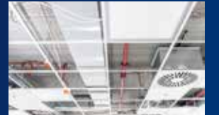
2 Cable inlets, ducts, lighting fixtures
